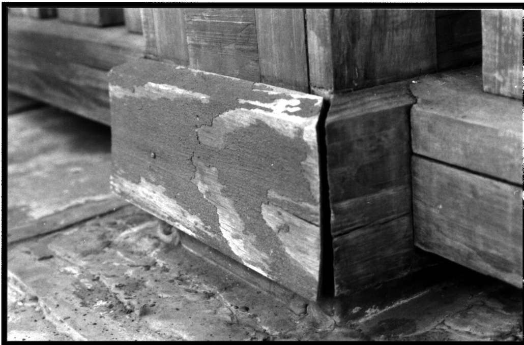
Figure 11. Only eight years after construction with new wood the base boards on this newel post are warped allowing water entry. Notice how paint has fallen off in the characteristic flame pattern indicating flat-grain wood.
