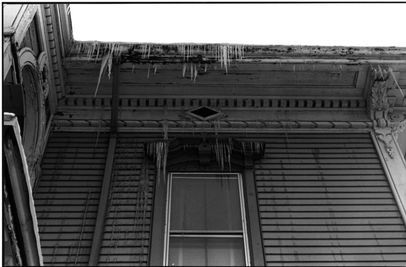
Figure 1. The cornice (top of photo) is damaged by water pouring over and through deteriorating gutters that leak due to decay.
